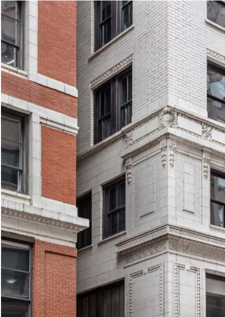
Below: some parts of the terracotta tiles have cracked or broken off. Rubber molds were used on existing ornaments to aid in making replacement copies.
